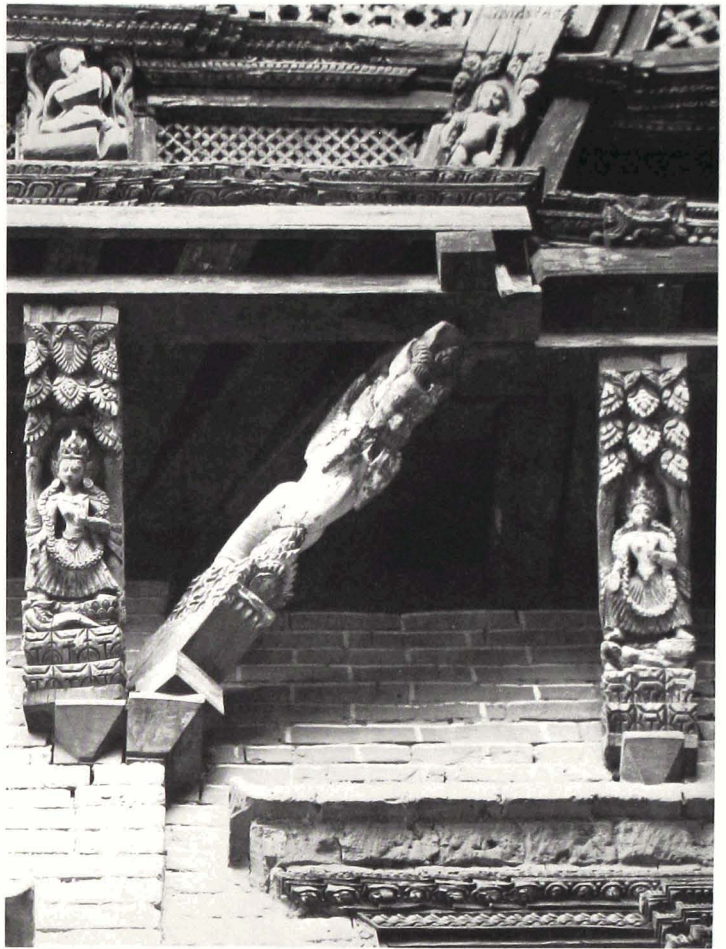
63 Sundari Chok, East Wing, Struts supporting Balcony
